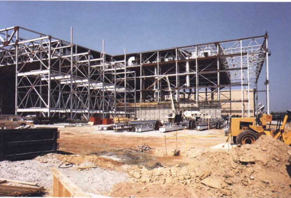
By meeting tight delivery deadlines, United McGill helped the contractors keep the project on schedule.
