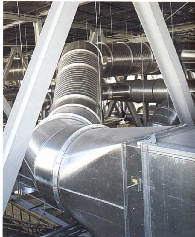
Engineering time was saved by using the UNI-DUCT® computer program to redesign the air handling system with round duct.
